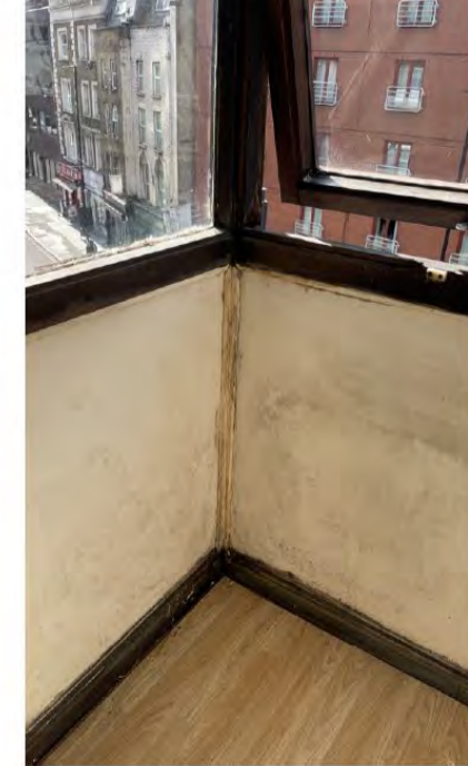
Paintwork deteriorating on timber frame and the spandrel panel. Evidence of mould growth.
