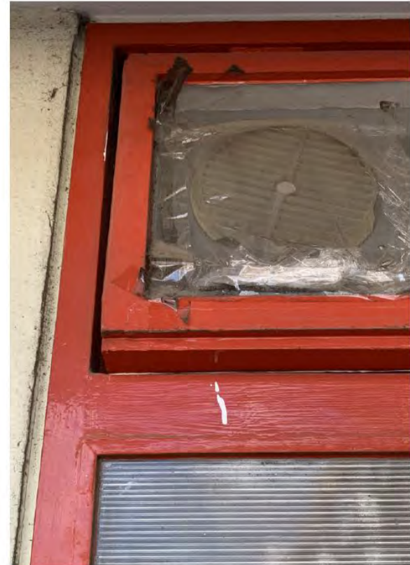
Ventilation panels have been retrofitted into some windows and some have subsequently been covered to stop any draughts.
