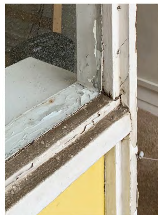
Paintwork deteriorating on timber frame/sill (internal and external).
