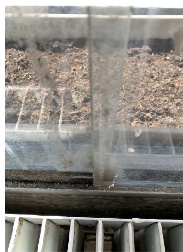
The original sliding aluminium bar appears to be missing on some of the unframed sliding windows, leaving a gap for warm to escape out of.
