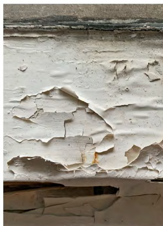
Paintwork deteriorating on timber frame/sill (internal). Evidence of mould growth.
