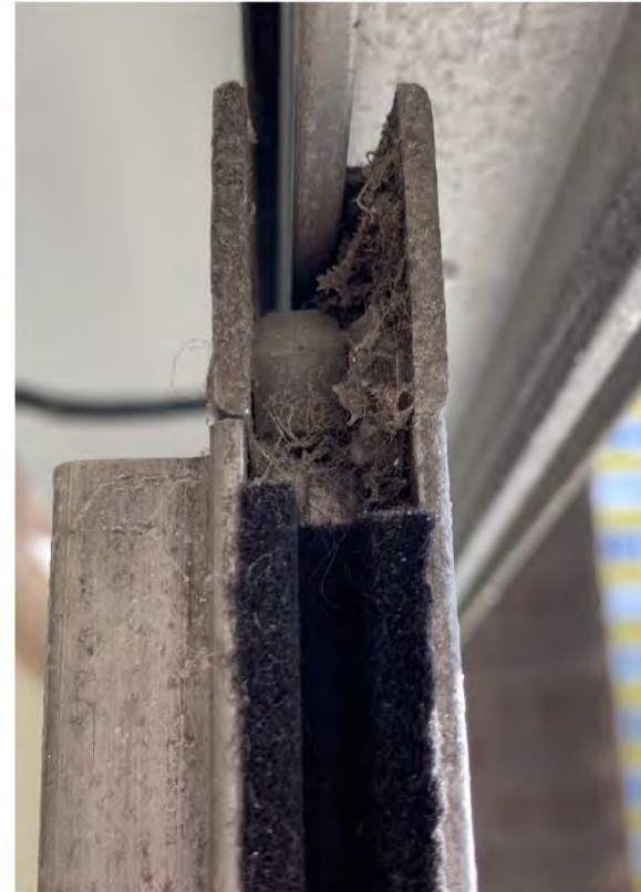
The original aluminium frames and runners are weathered and stiff, showing signs of oxidation.
