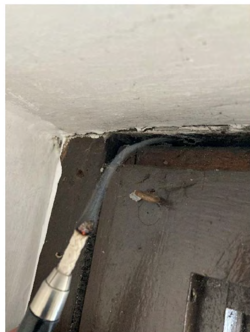
Photograph 14: Air Leakage - window frame (SAL12)
