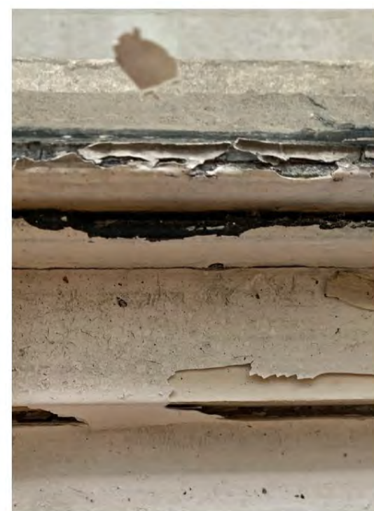
Paintwork deteriorating on timber frame/sill and steel opening lights (internal).
