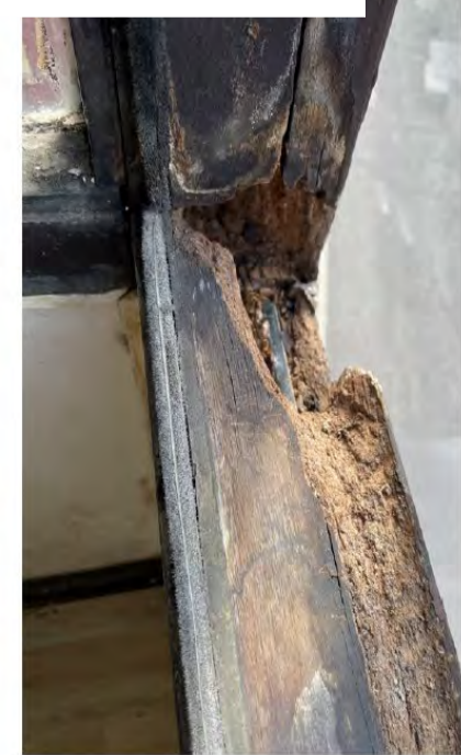
Deterioration of the hardwood frame/sill on the west facade (oriel window).
