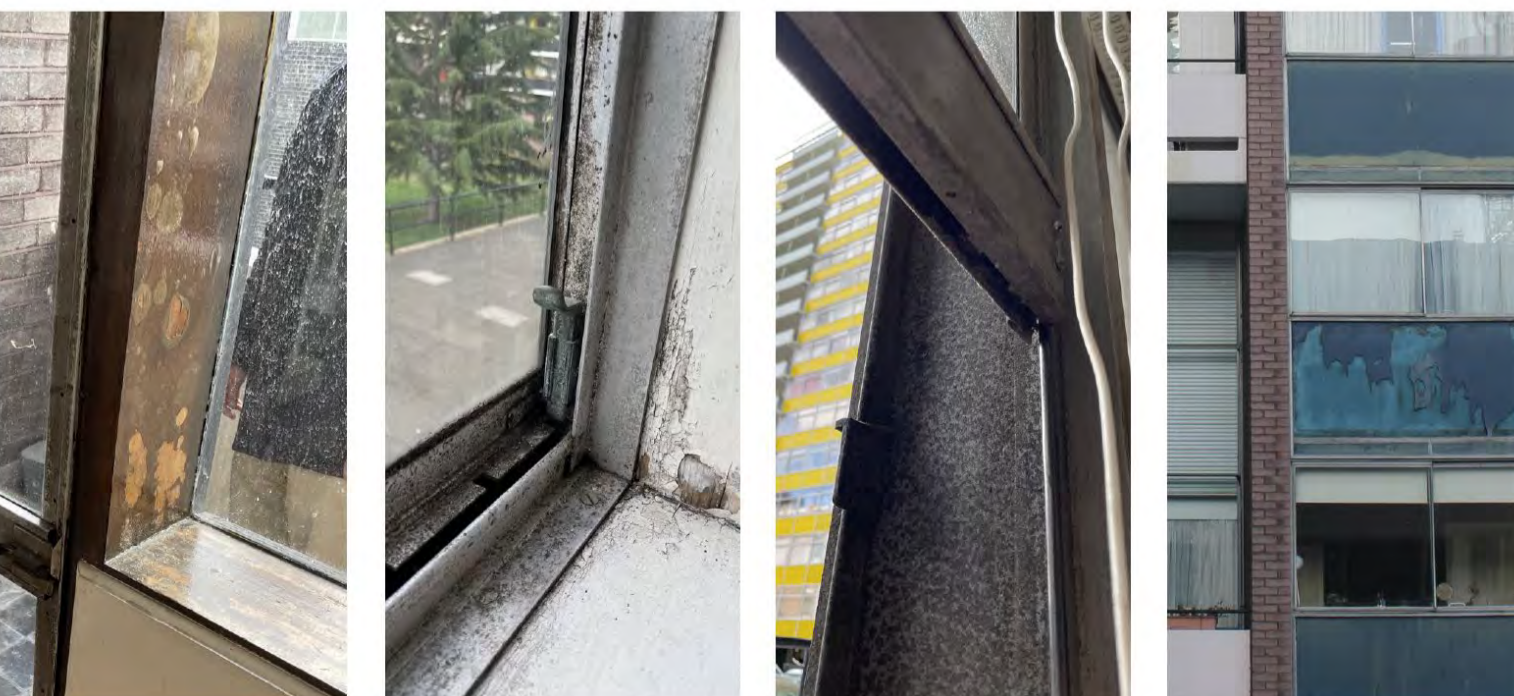
Protective coating on timber frame Oxidisation of the aluminium frames internally and externally (sliding). Peeling paintwork to timber reveal Oxidisation of the aluminium frames internally and externally (door system) Damage/deterioration of the Miroglass spandrel panels. Many are faded or have been replaced with a poor colour match
