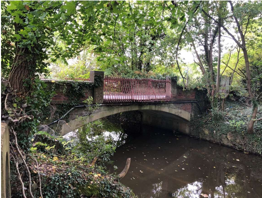
Figure 3 Dense vegetation growth, view from South-eastern side of the bridge
