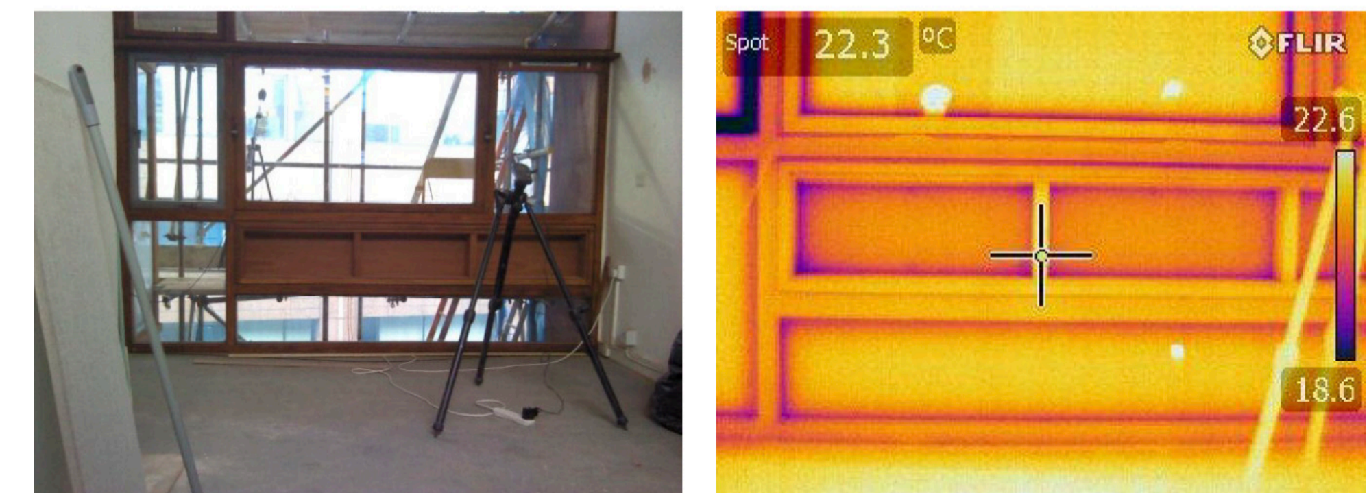
Figure 21: Thermal Image shelving minimal heat loss highlighted Location THL5 (see figure 7)
