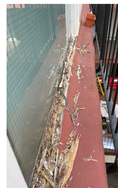
Deterioration of the softwood frame/cill on the kitchen window facing the internal lightwells.
