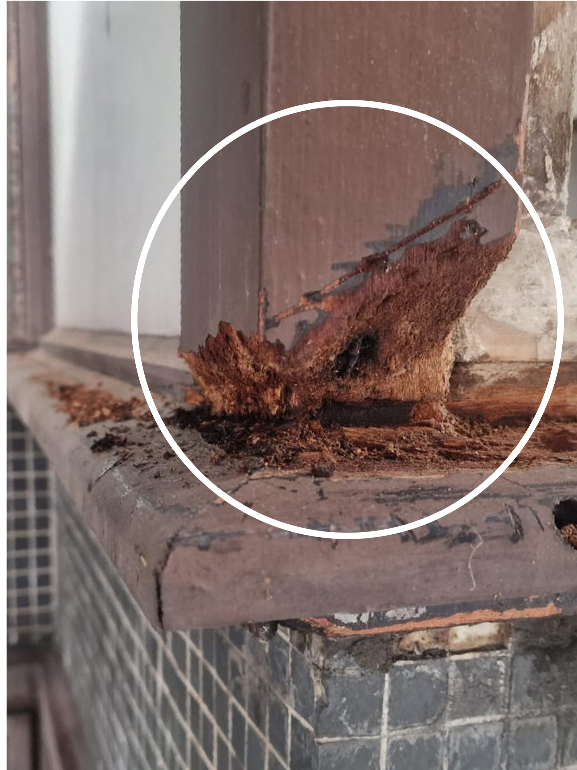
This photos shows the corner post after the rotten timber has been removed.
