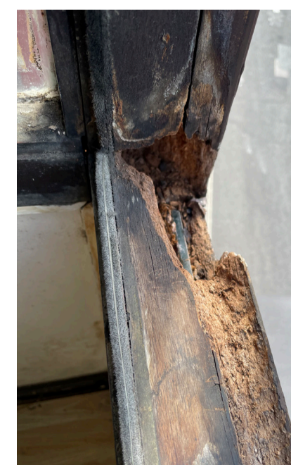
Deterioration of the hardwood frame on the west façade (oriel window).
