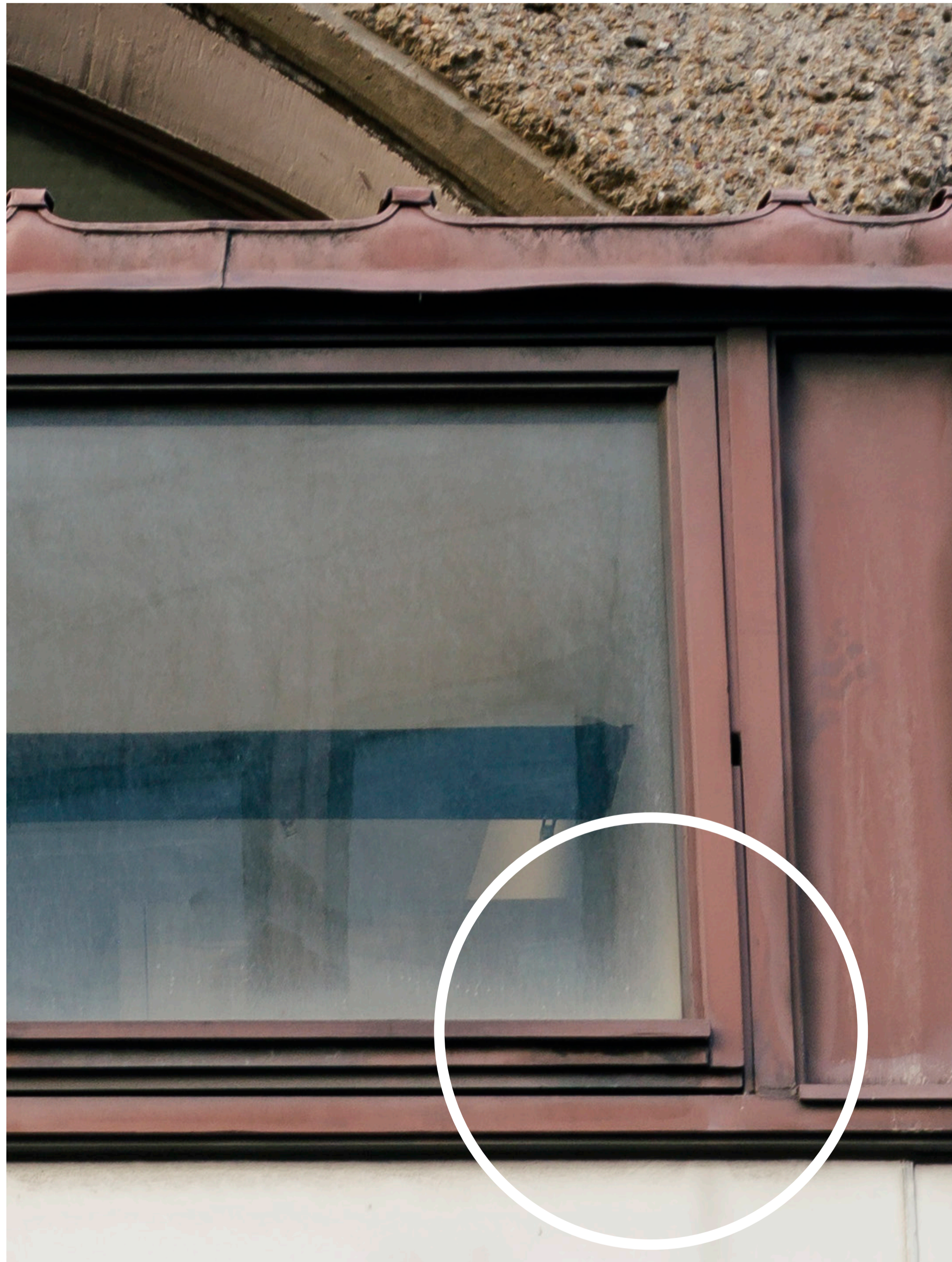
The same corner joint is shown in each of these three photographs. This photo shows the window frame prior to starting the Pilot Project and there is no obvious visible rotten timber.
