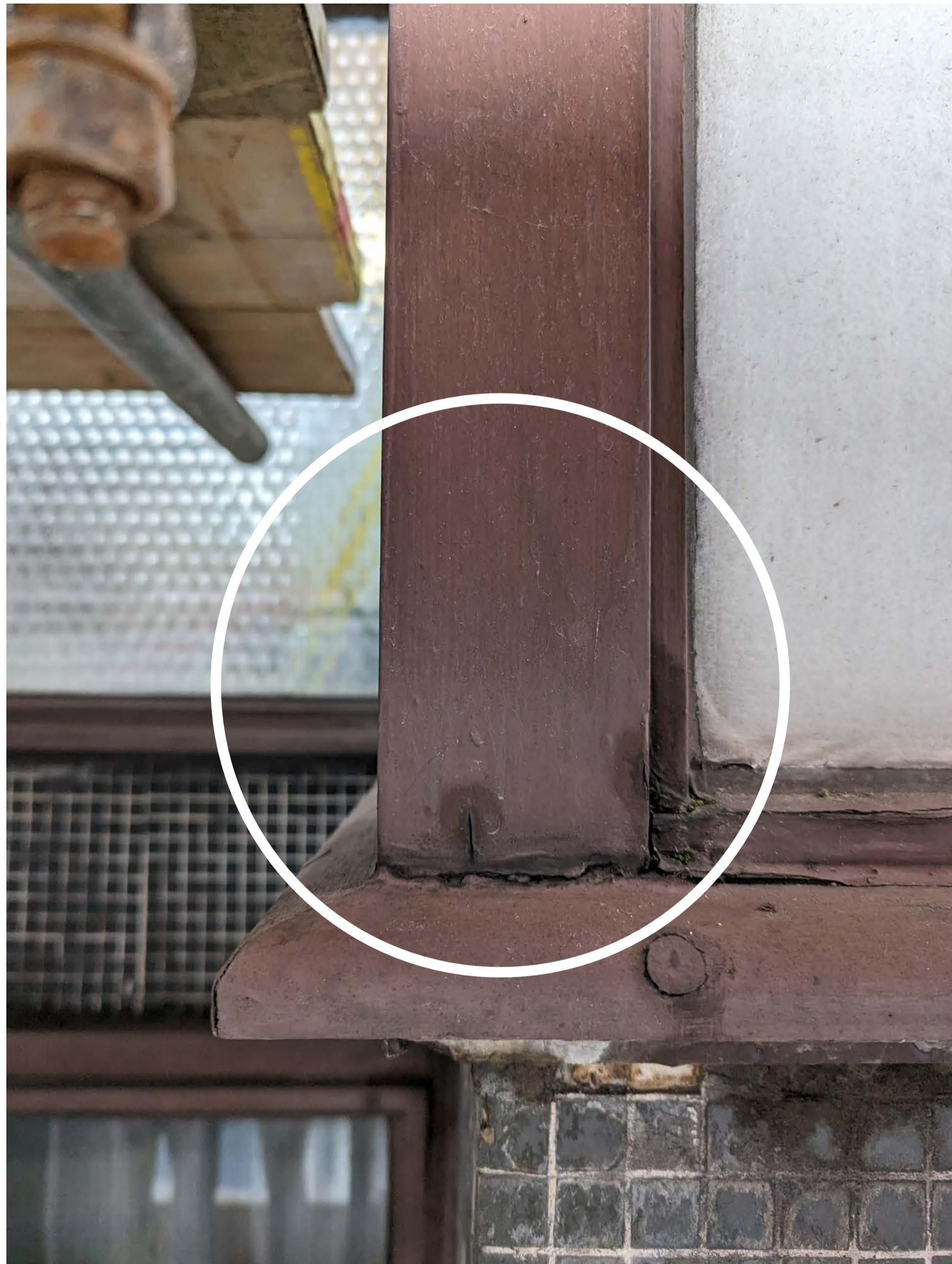
The same frame joint is shown in each of these three photographs. This photo shows the corner post of the window frame prior to starting the Pilot Project and there is no obvious visible rotten timber.
