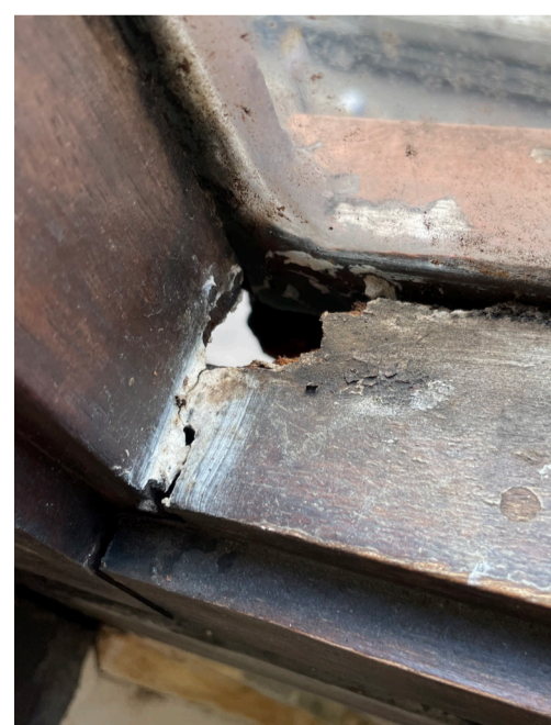
Deterioration of the hardwood frame/cill on the west façade where the glass pane has become exposed to the elements. Evidence of mould growth.
