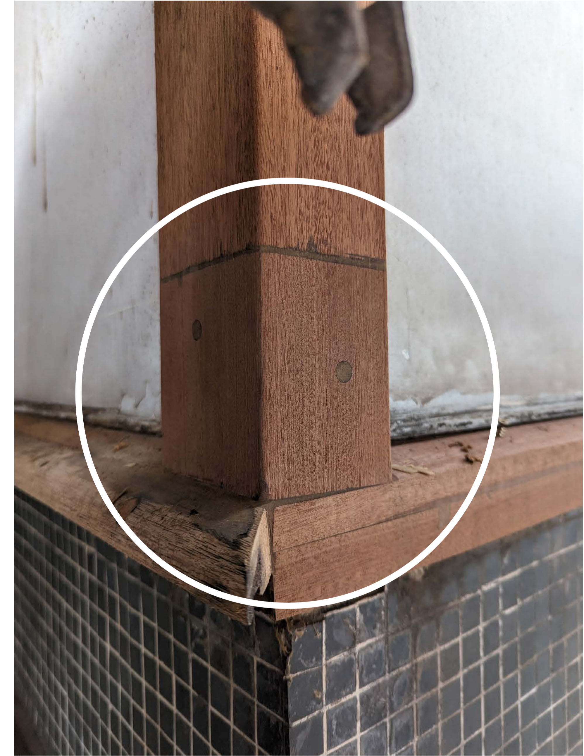
This photo shows the repaired post (before final finish applied) with new sapele spliced into frame, spliced timber mechanically fastened to existing frame and resined in place.
