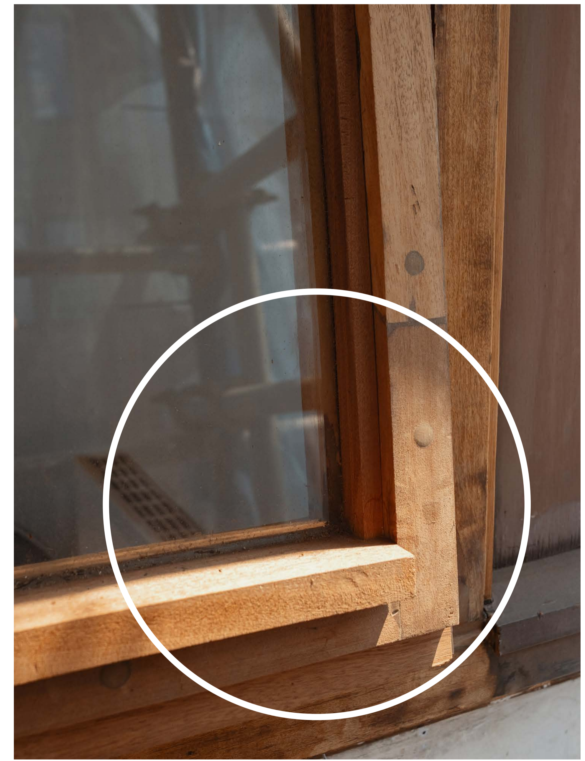
This photo shows the repaired frame (before final finish applied) with new sapele spliced into frame, spliced timber mechanically fastened to existing frame and resined in place.
