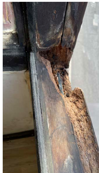
Deterioration of the hardwood frame/sill on the west façade (oriel window).
