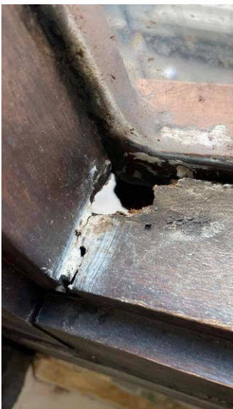
Deterioration of the hardwood frame/sill on the west façade where the glass pane has become exposed to the elements. Evidence of mould growth.
