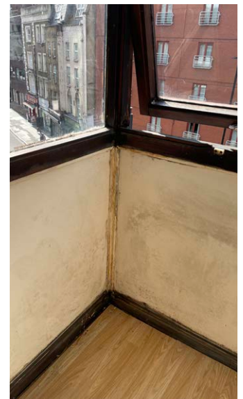
Paintwork deteriorating on timber frame and the spandrel panel. Evidence of mould growth.
