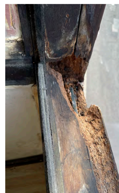
Deterioration of the hardwood frame/vv on the west façade (oriel window).
