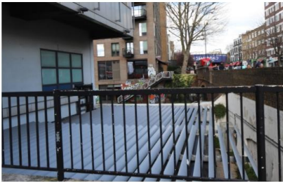
(C) Unsightly louvre over the plant space adjacent the listed bridge, Camden Road
